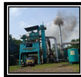
Gambar 2. Asphalt Mixing Plant
