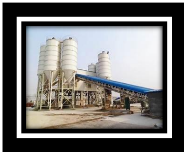
Gambar 3. Concrete Batching Plant Sumber: Goggle
